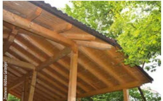
Carport without brace.
